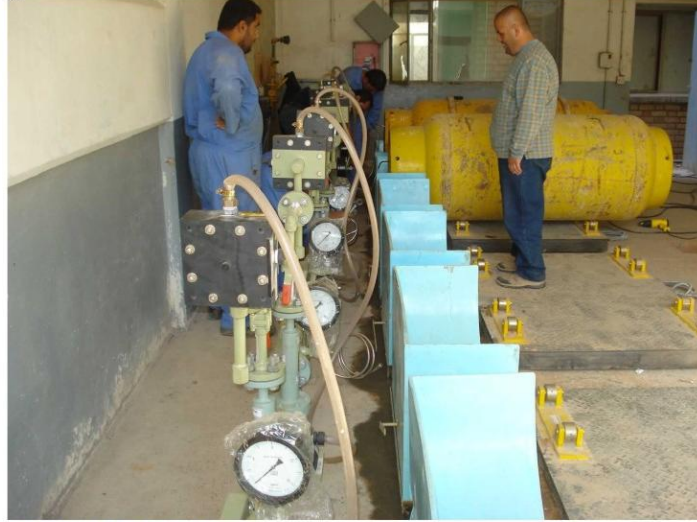
Line-III, chlorine unit
